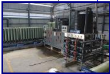
BMSW RO PLANT
