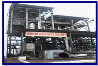
BMSW EVAPORATOR-II & ATFD
