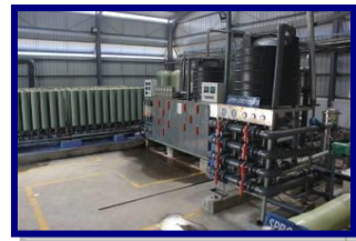
BMSW RO PLANT
